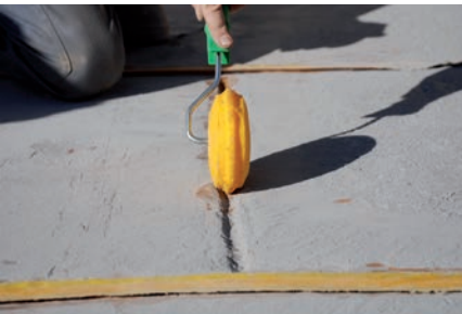
Repaso de juntas con roler o taco. Going over with roller or block.
